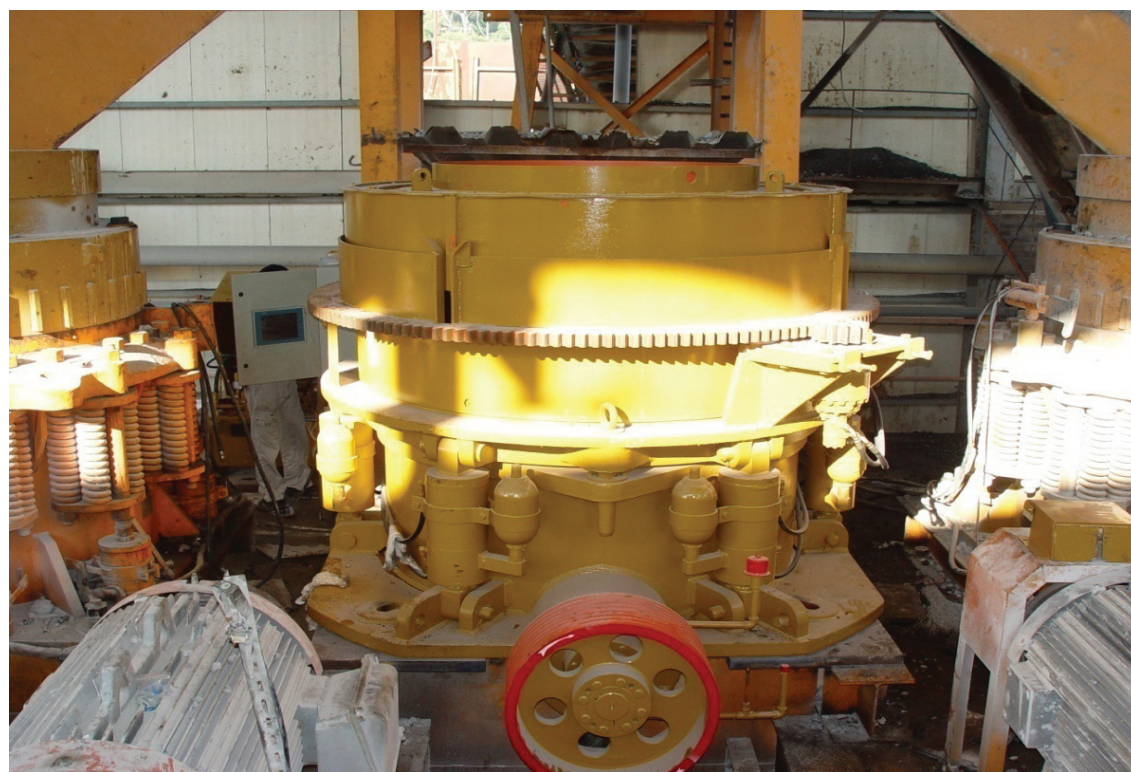
Cone Crusher MSC400, 400 TPH, at a quarry in Central Taiwan
