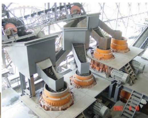
Cone Crusher 400TPH in Central Taiwan.
