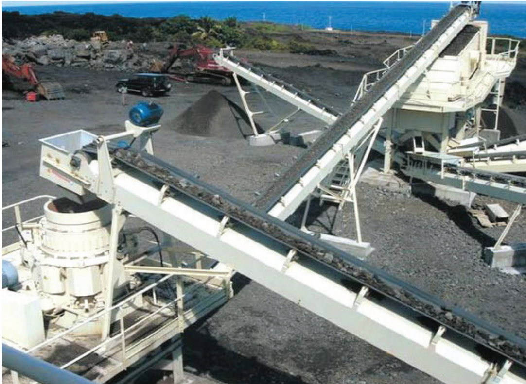
Crushing & Screening Plant at 100TPH Throughput in Morocco.
