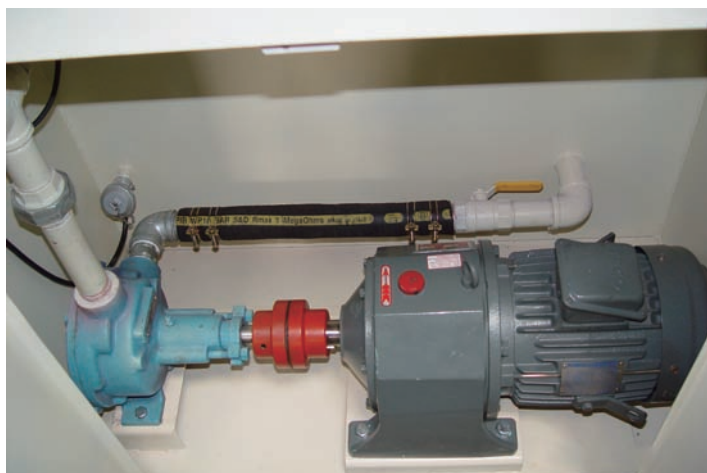
Safety Device of Lubrication System
